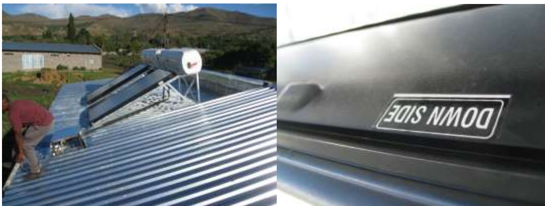
Figure 2: Poor positioning of the collector ( Source: Rudi Moschik, AEE-Institute for Sustainable Technologies).
