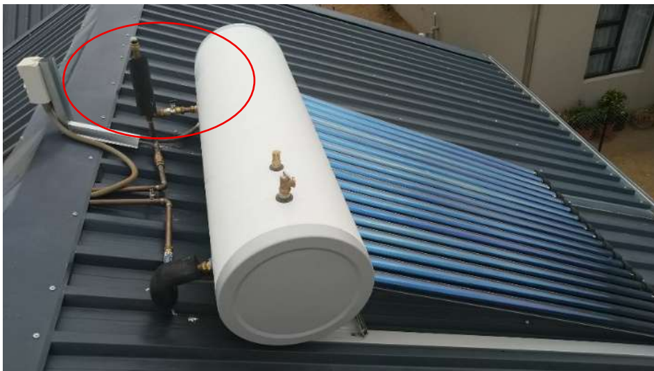
Figure 3: Wrong positioning / installation of vacuum breaker.
