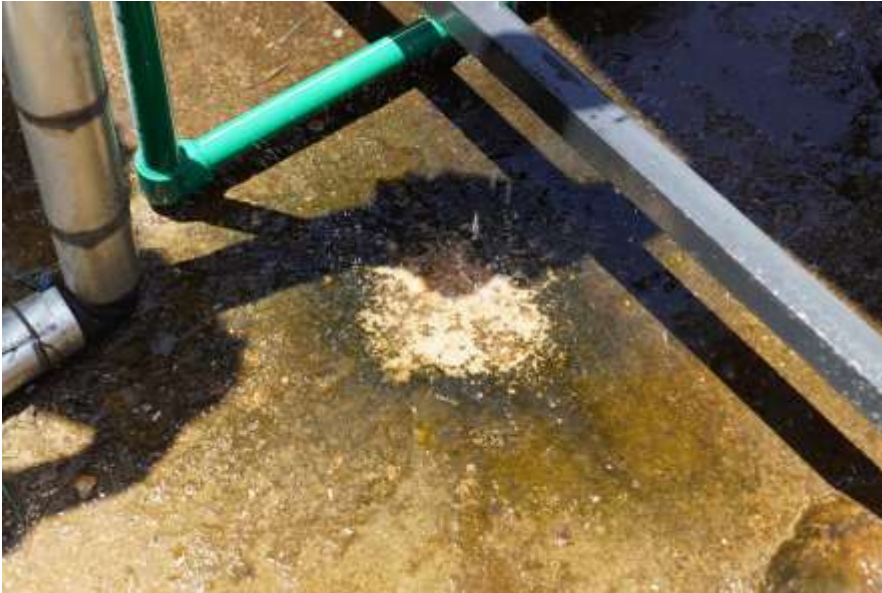
Figure 9: Consequences of the leak ( Source: Rudi Moschik, AEE-Institute for Sustainable Technologies).
