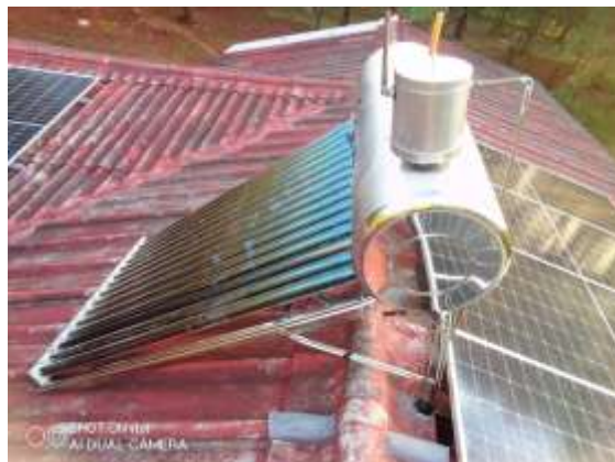
Figure 1: Wrong way of installation of solar geyser would lead to roof breaking.
