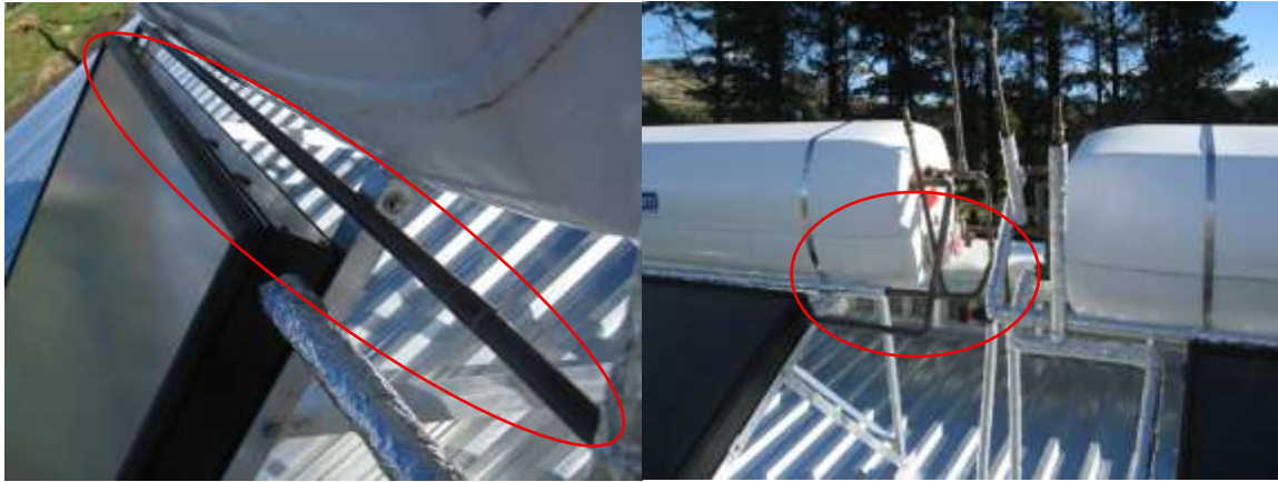
Figure 5: Missing insulation protection ( Source: Rudi Moschik, AEE-Institute for Sustainable Technologies).
