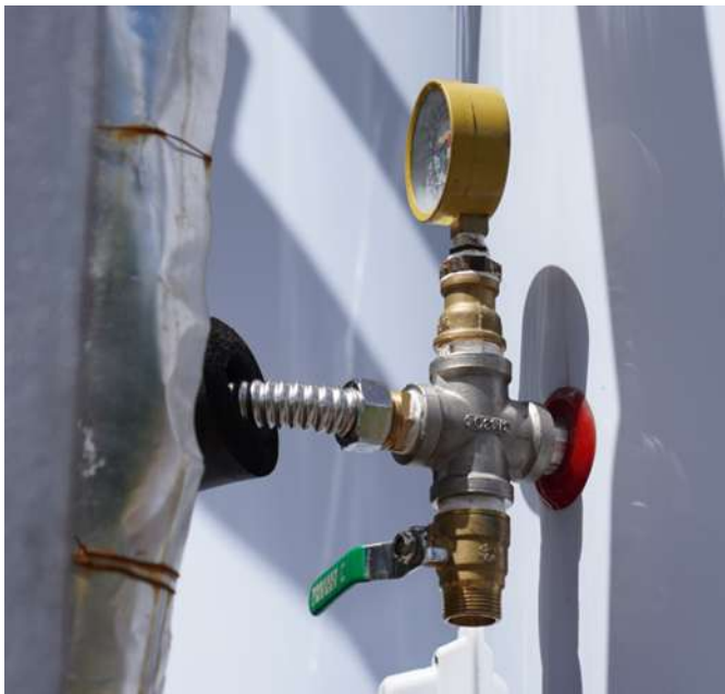
Figure 7: Missing safety devices. ( Source: Rudi Moschik, AEE-Institute for Sustainable Technologies).
